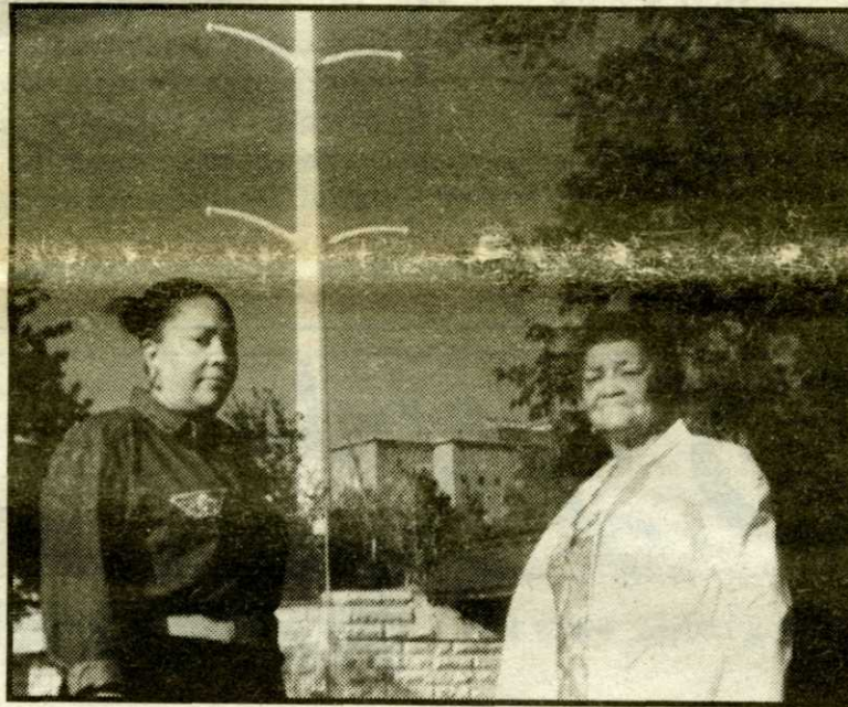
Ceila Butler and Arlene Arikpo of the Washington Park Community Coalition stand in the foreground of a power on 55th and Federal Commonwealth Edison is constructing.
