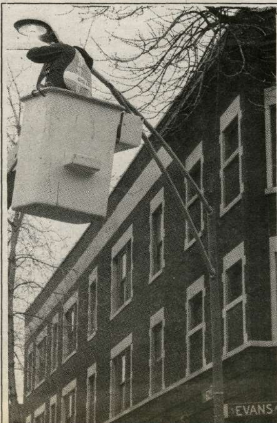
This vandalized street light at the corner of 62nd & Evans was repaired recently by Streets & Sanitation electricity bureau workers. Commissioner Eileen Carey urged local residents to report non-functioning street or alley lights immediately to City Hall's 24-hour service request line at 744-5000.
